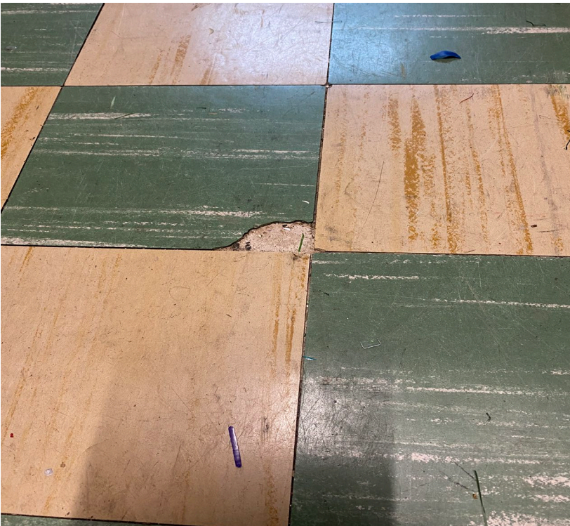
Damage shown in tile. This was not evident in the 2016 inspection. (Original photograph available on Page 73 of the Asbestos survey).
